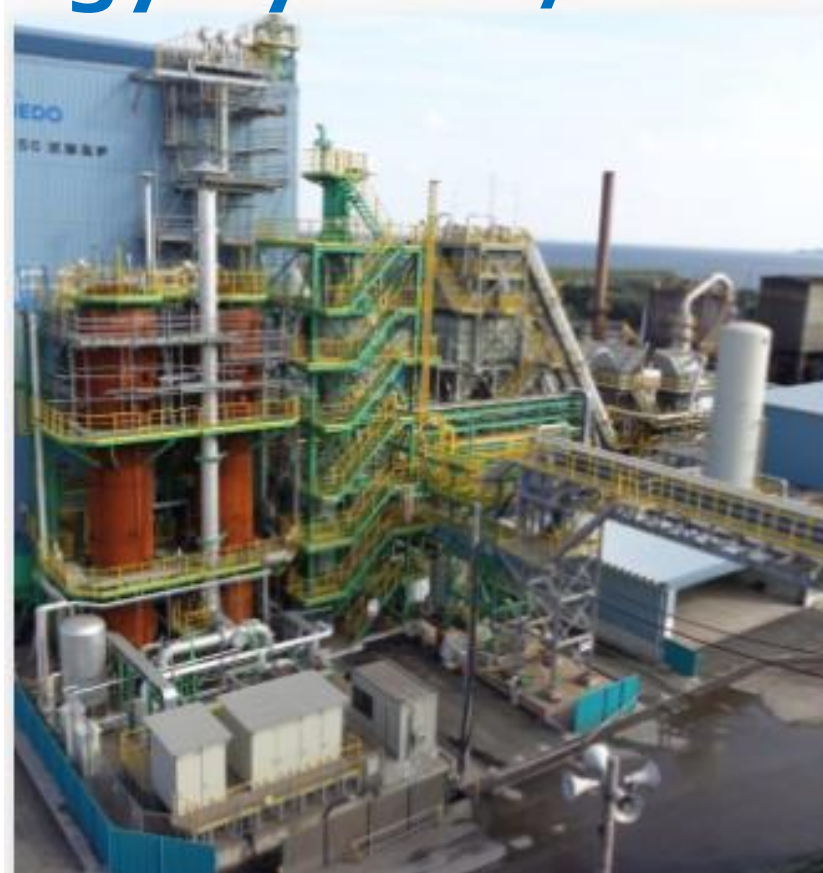
【Photo】 Experimental/demonstration Furnace by a consortiums composed of iron/steel manufacturers and NEDO (@Kimitsu) (Source : Iron and Steel Association of Japan HP)
